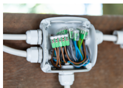
Wiring in the distribution box
